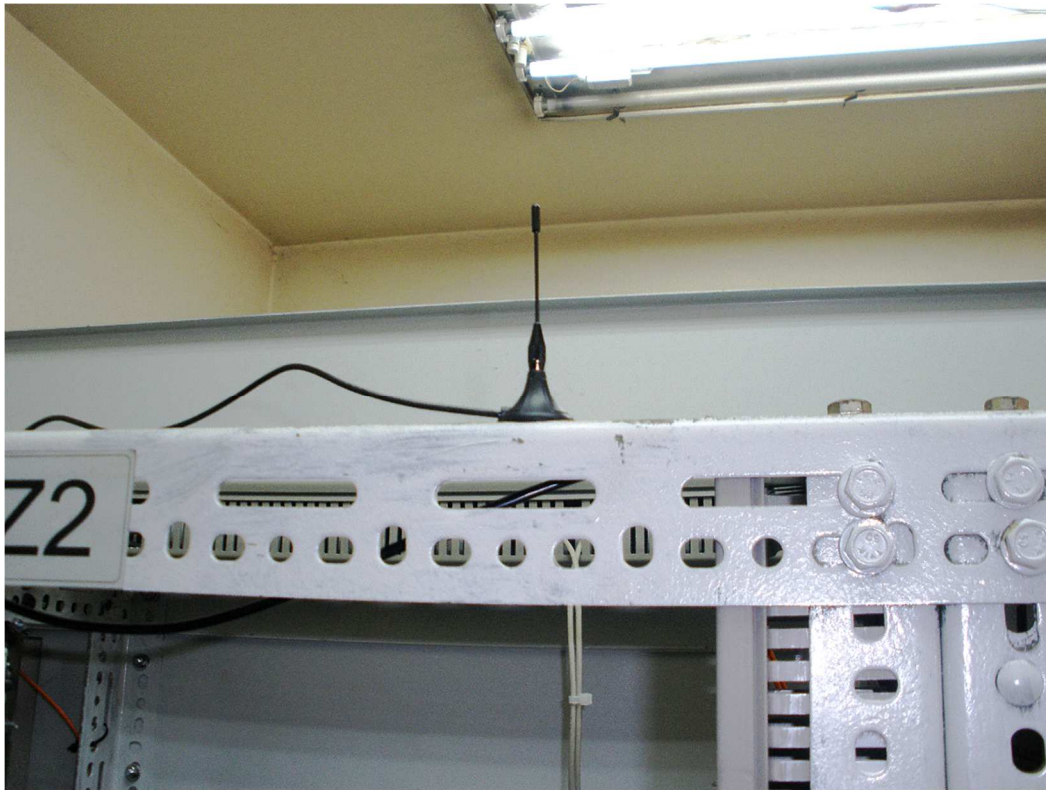
Fig. 13. STER PMU installation – GPRS antenna with magnetic support
